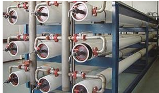
Reverse osmosis system
